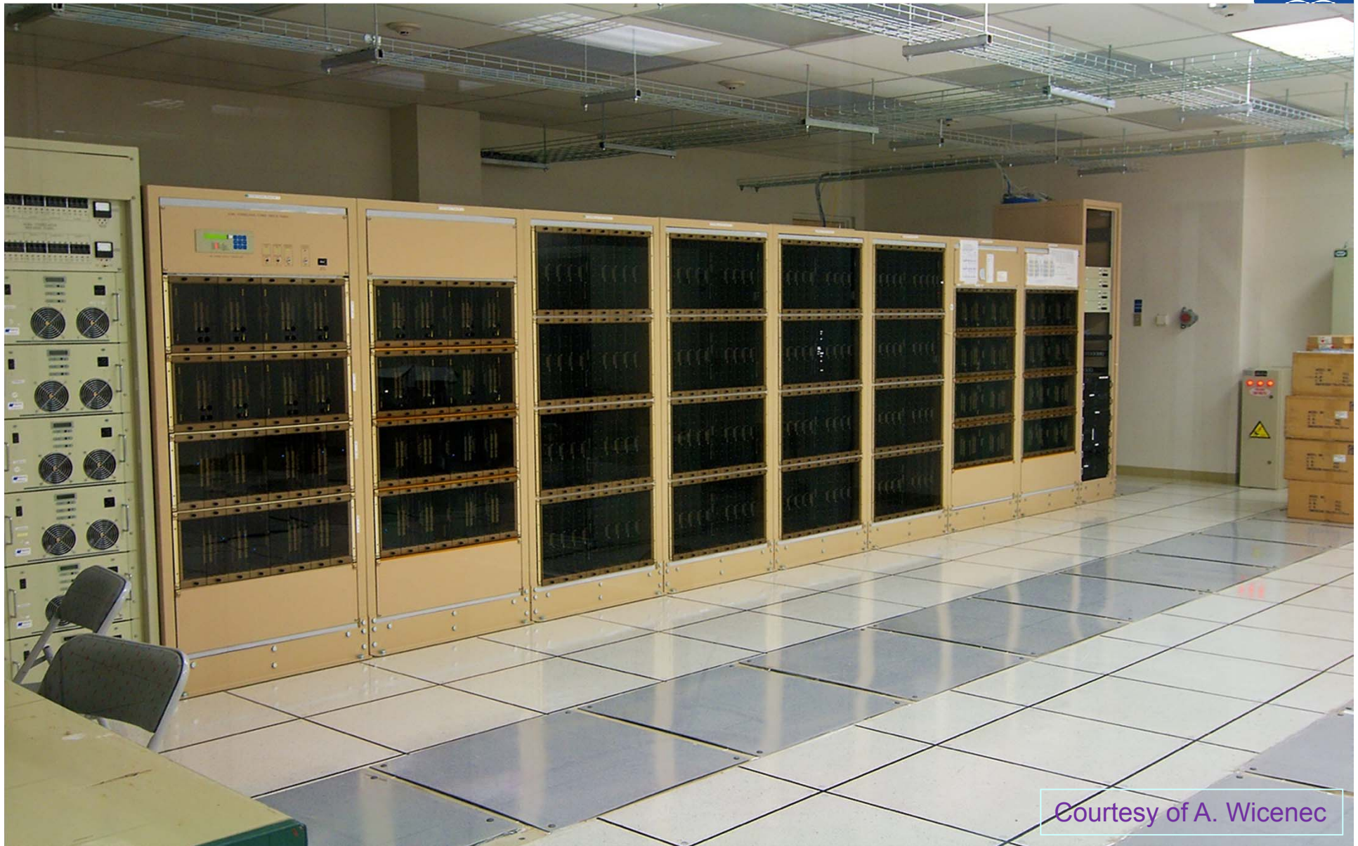
FPGA based correlator: Highly customized HPC system directly attached to antenna output. Image shows one quadrant of ALMA correlator installed on the Chajnantor plateau (Chile) in 5000m elevation. Image: A. Wicnec
